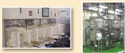
Wafer cleaning equipment Chemical supply system
